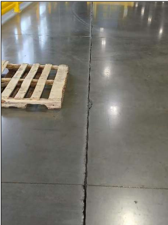
Photo 4: Photo of a gap in caulk along concrete seam in the southwest corner of the warehouse.
