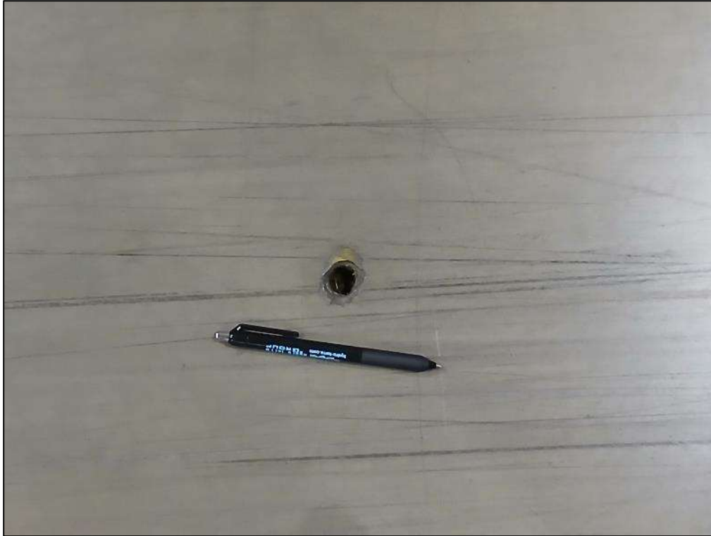
Photo 3: Photo of a small hole in the concrete near AD238.
