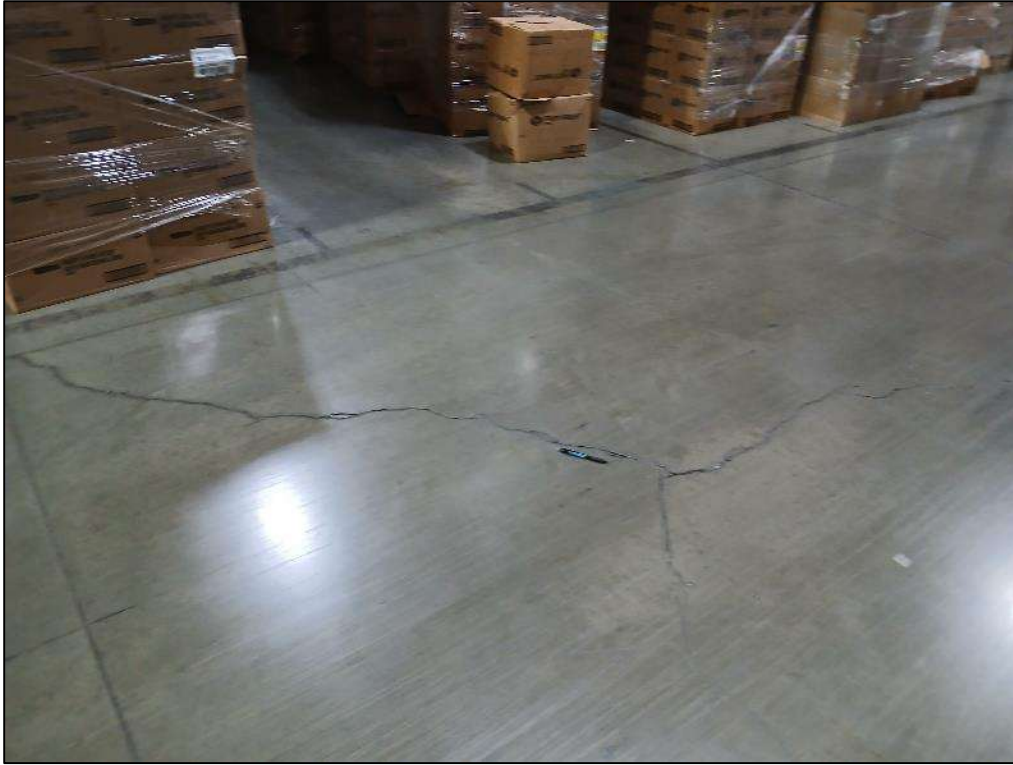
Photo 1: Photo of cracks in the concrete near location G227.
